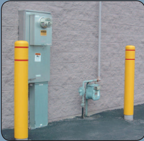
Figure 1: Two Pipe Bollard covers stationed near a building's exterior junction box
